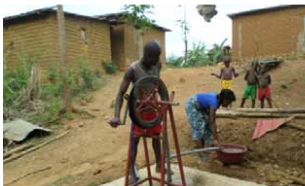
Rope pump installed. Right now there are 13 pumps installed in the gardens for irrigation and pumps installed in 4 locations for water supply for domestic use, FC Cabinda.
