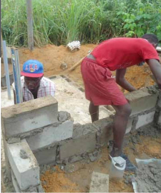
Water Assistants from EPP Cabinda students constructing latrins at the community pre-school.
